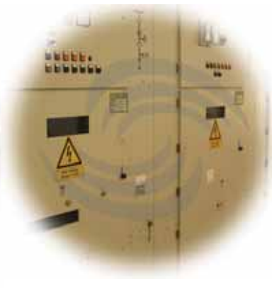
Indoor 33KV switch gear panels
